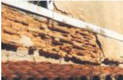
Venice: salt damage to brickwork and plaster.
